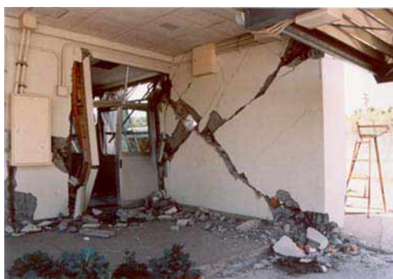
Damage class V
