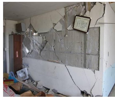
Figure 11. Shear failure in shear wall
