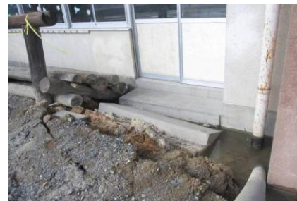
Figure 25. Liquefaction evidence located 3 stair steps from the ground surface.
