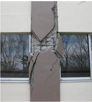
Figure 16. Shear failure in column
