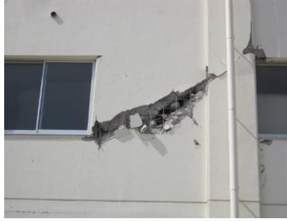
Figure 20. Shear failure in wing wall
