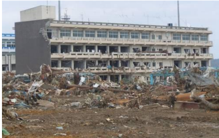
Figure 26. Flood reached 3 rd floor
