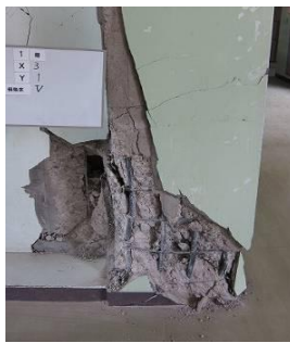
Figure 10. Shear failure in column
