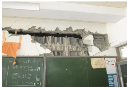
Figure 23. Partial collapse of concrete blocks partition wall
