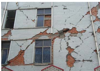
Fig. 1 Damage of RC building with masonry infill in China 2008 Wenchuan earthquake
