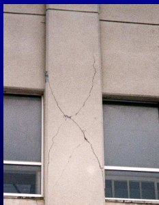
Crack width of 2mm
