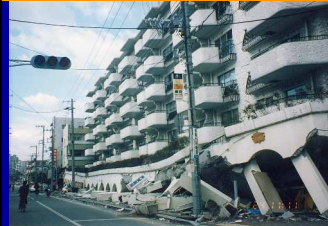
Story collapse (1995 Kobe EQ)
