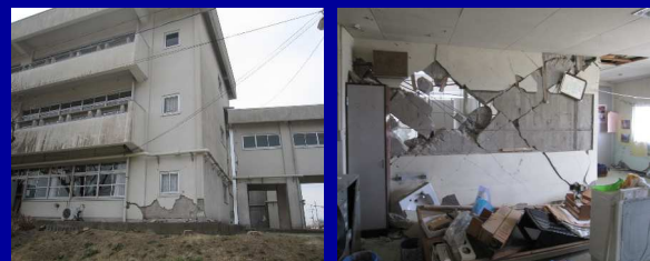
Severely damaged school building (Shitigahama town) Shear failure of RC wall
