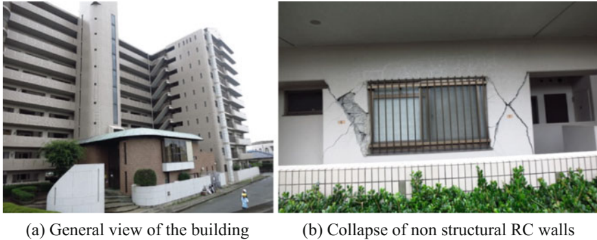
Fig. 11 Damage to a residential building in 2016 Kumamoto Earthquake
