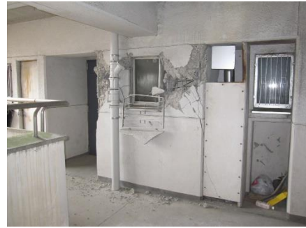
b) Damage to non-structural RC walls
