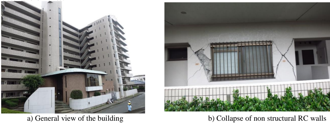
Fig.11 - Damage to a residential building in 2016 Kumamoto Earthquake
