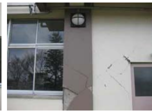
Fig.16 Shear Crack in side walls. Building (W)
