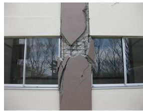
Fig15. Shear failure in column. Building (W)
